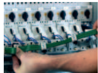
Fault-free mounting and wiring
